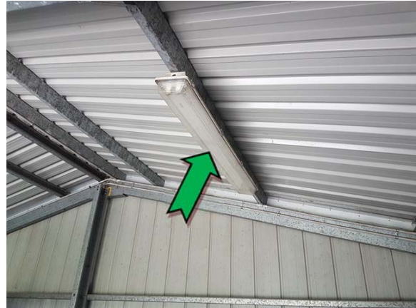
Photo 2. Interior, throughout, double tubed fluorescent light fitting – suspected non PCB-containing capacitor.
