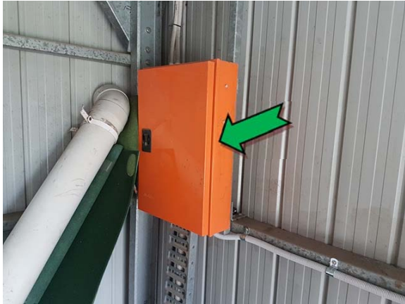
Photo 1. Interior, west elevation, electrical backing board – suspected non asbestos-containing bituminous backing board.
